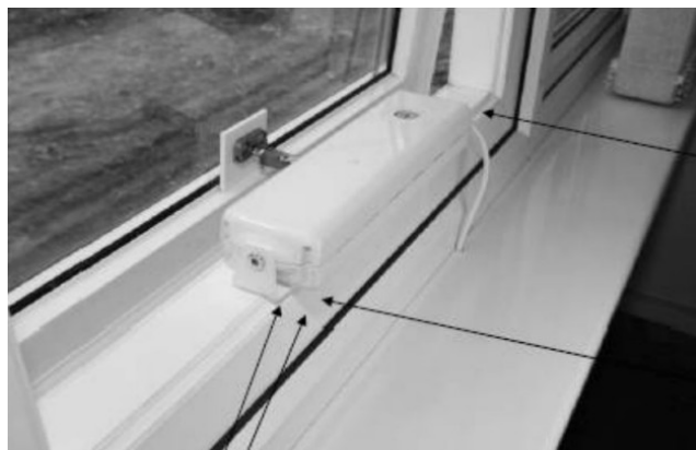
Roof vent shown fitted vertically for test purposes
